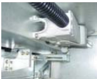
Withdrawable circuit breaker control wiring plug&socket
