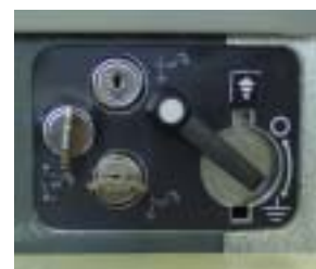
Interlocks on earthing switch operating mechanism
